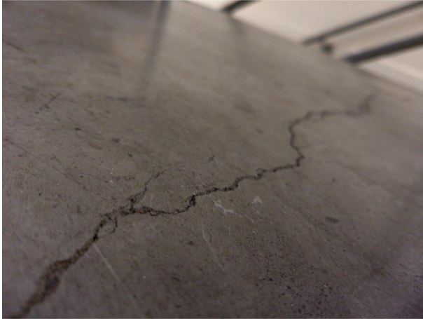
A crack in the concrete of the Clark Hall stairwell. Jaron Kent-Dobias, unpublished (2019).
